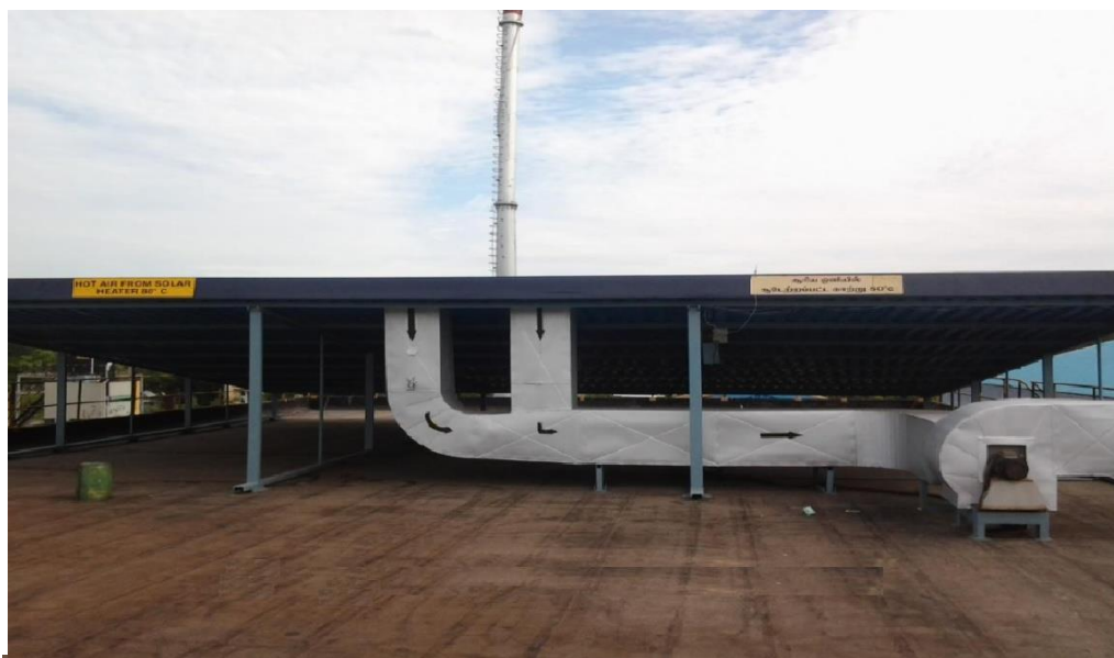
Plate 6.1. A view of Solar Air Dryer
