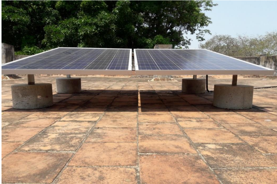
Figure 2.23: Front View Of Solar Panel
