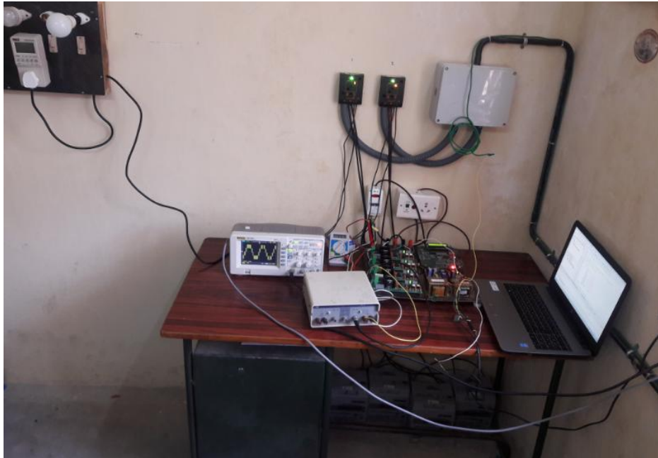
Figure 2.27: Photograph of Cascaded Multi Level Inverter Interfaced with PV resource in the EEE Department of PEC
