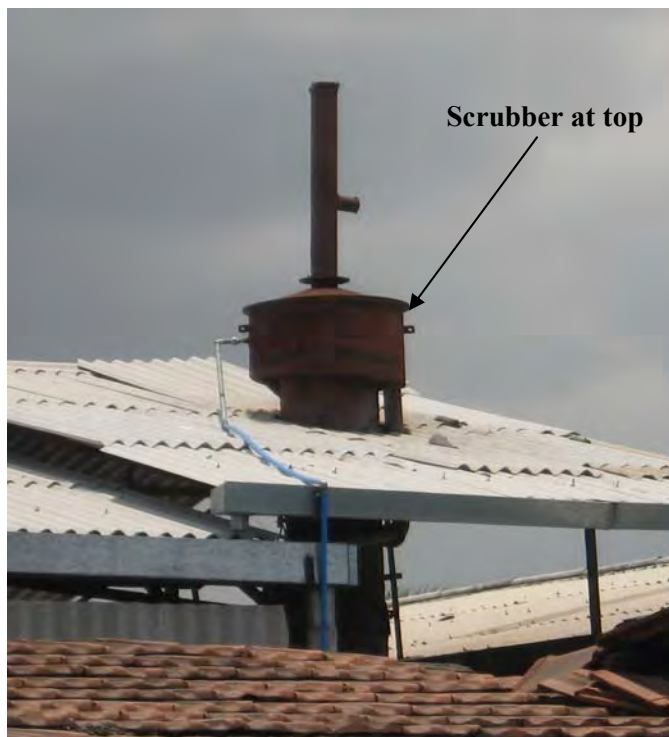
Figure 3-9: Low Cost Scrubber
