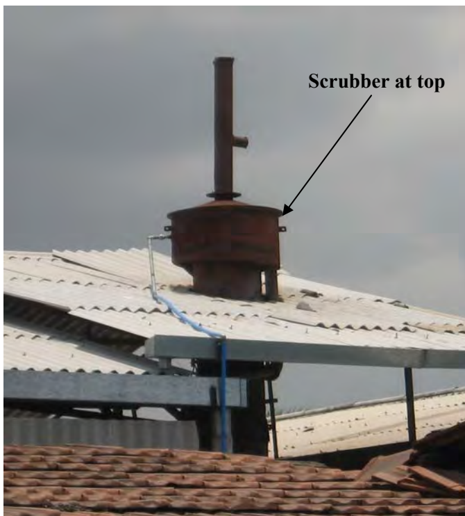
Figure 3-9: Low Cost Scrubber
