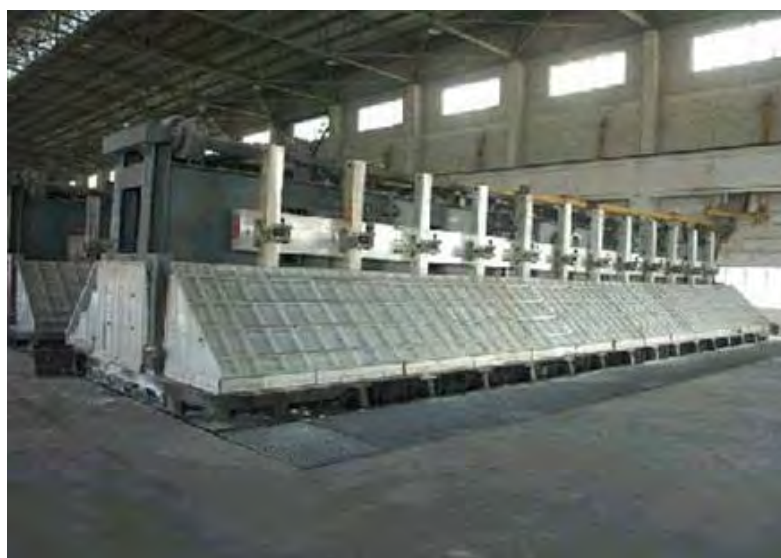
Figure 3-17: Electrolytic Cell for 300 kA Prebaked Carbon Anode Technology in the Cell Room
